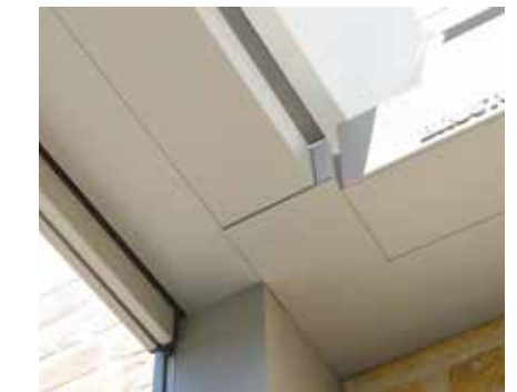
Waterafvoer via goot direct in steunpaal
