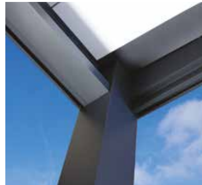
Waterafvoer via goot direct in steunpaal
